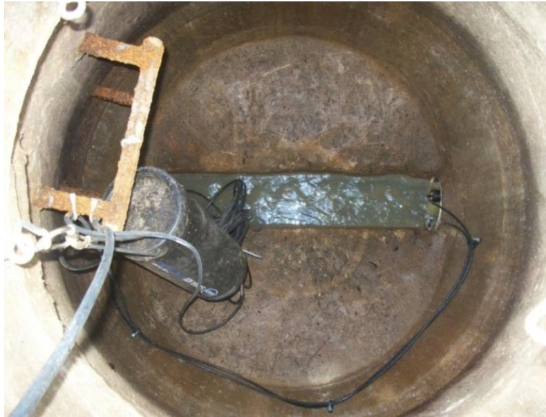
Photograph 1. Typical Flow Meter Installation
